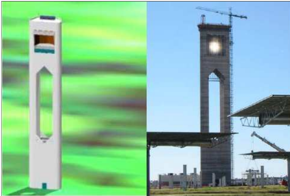
Figure 3-9: Tower of PS10 /FTPR 2005/
