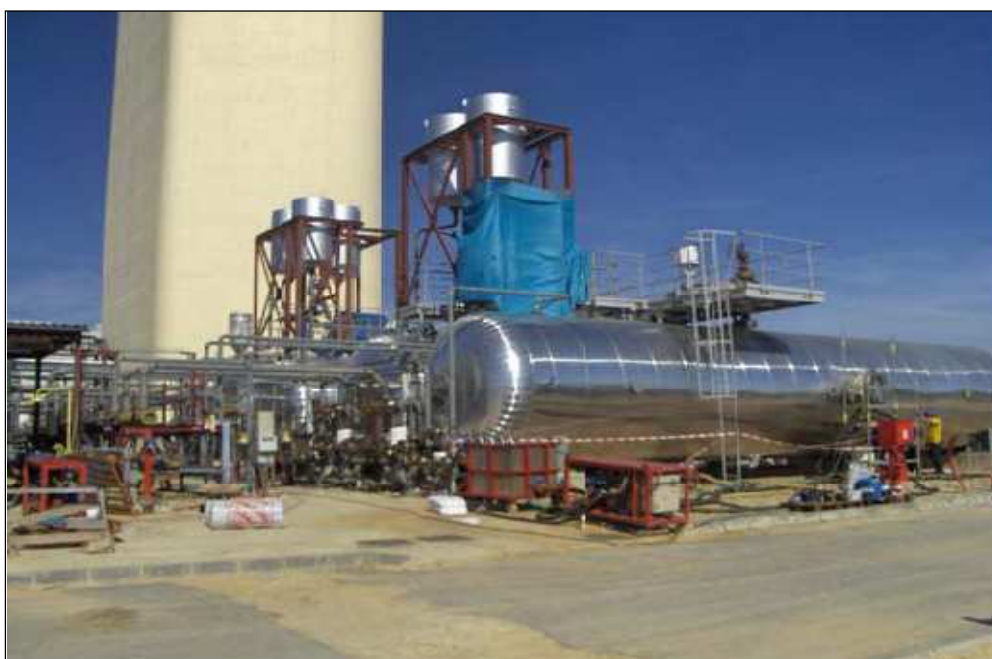
Figure 3-10: Thermal storage tanks of PS 10 /FTPR 2005/
